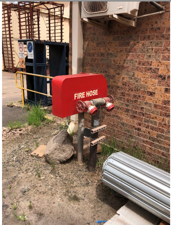
Picture 60: IMG_5955 Fire hydrant and hose reel
