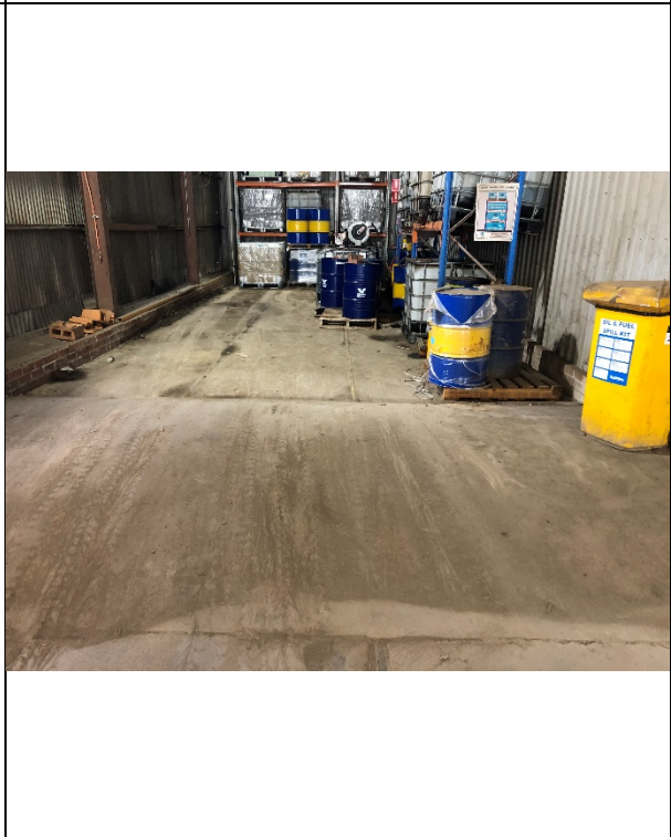
Picture 64: IMG_5960 Bunded oil and chemical storage
