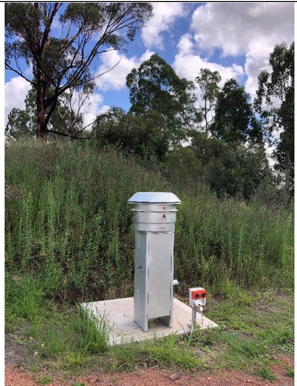
Picture 24: IMG_5899 Weather station adjacent to Dam 4
