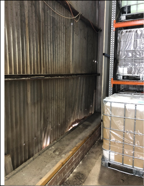
Picture 65: IMG_5961 Bunded oil and chemical storage
