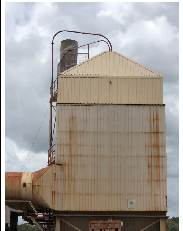
Picture 55: IMG_5949 Stack air emissions monitoring point
